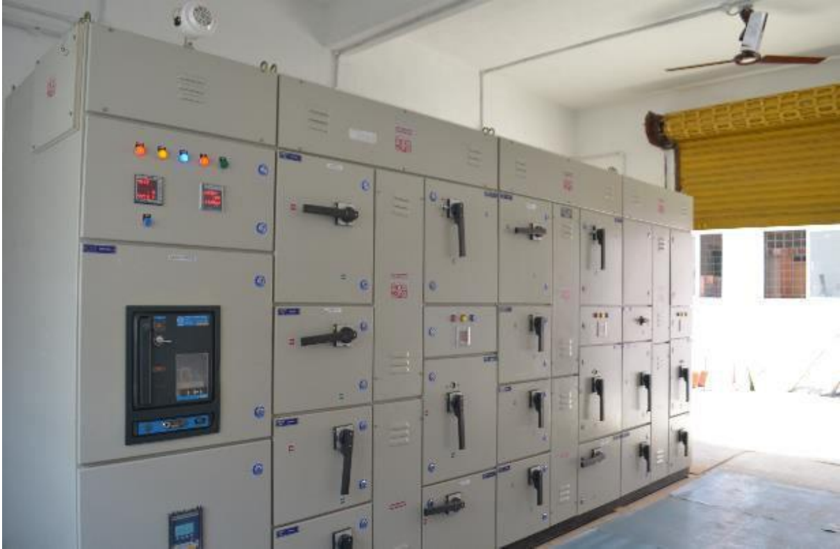
HT Substation Control Room
