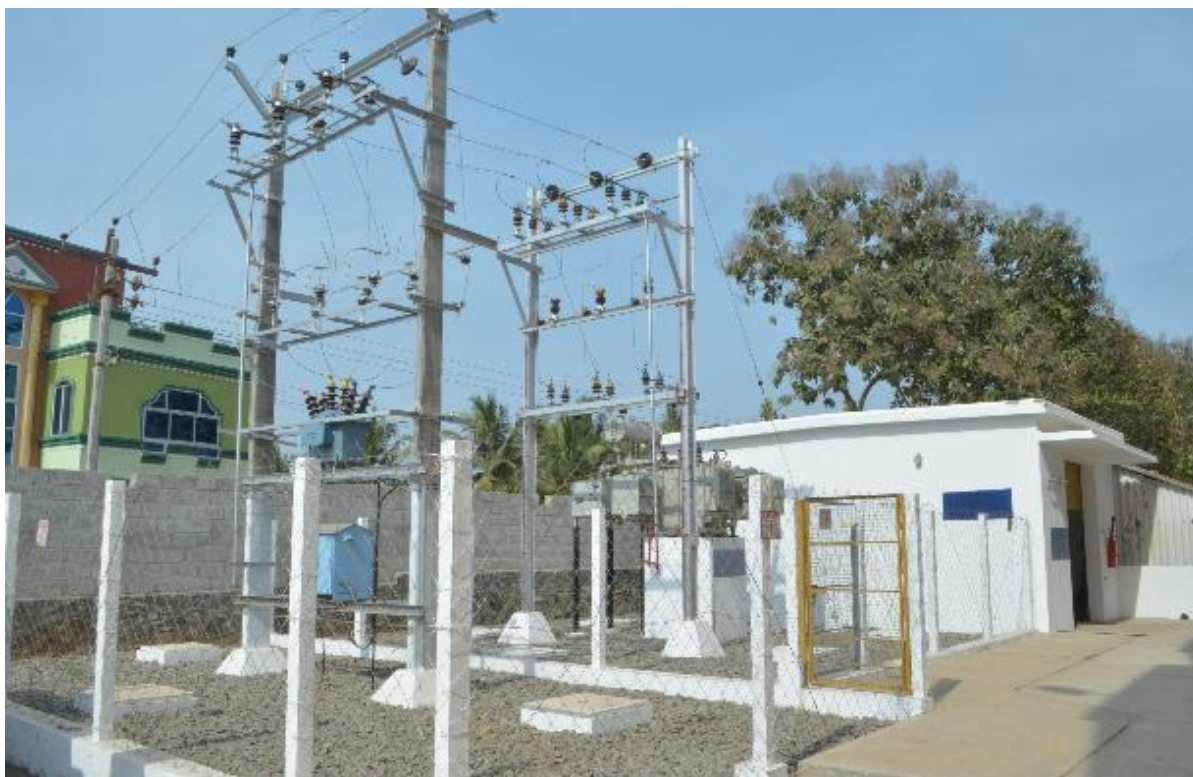
11 kV/415 V HT Substation
