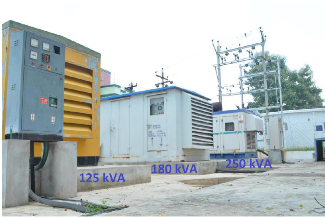
Kirloskar Diesel Generator (3Nos) installed in our College Campus for Backup Electric Supply
