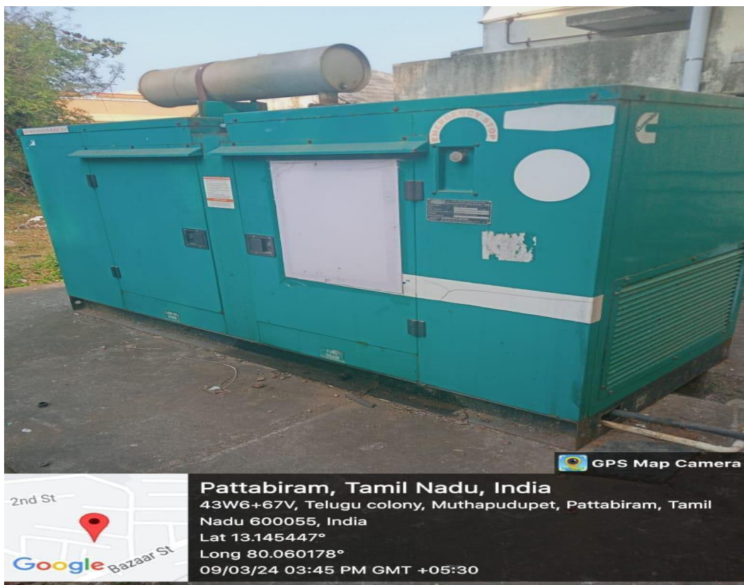
40 kVA Powerica Diesel Generator (1No) installed in our College Campus for Backup Electric Supply
