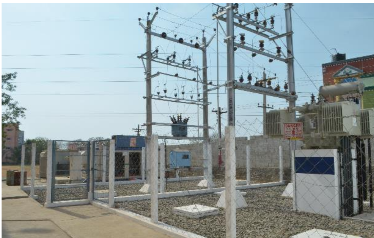
11 kV/415 V HT Substation
