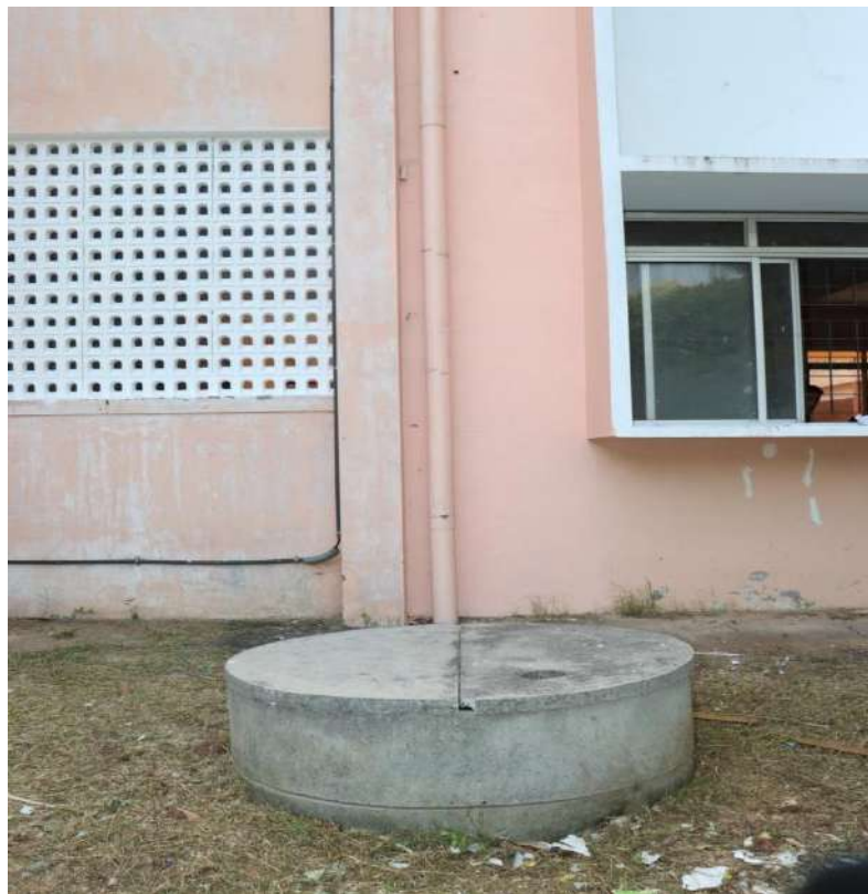
Recharge pit on campus grounds
