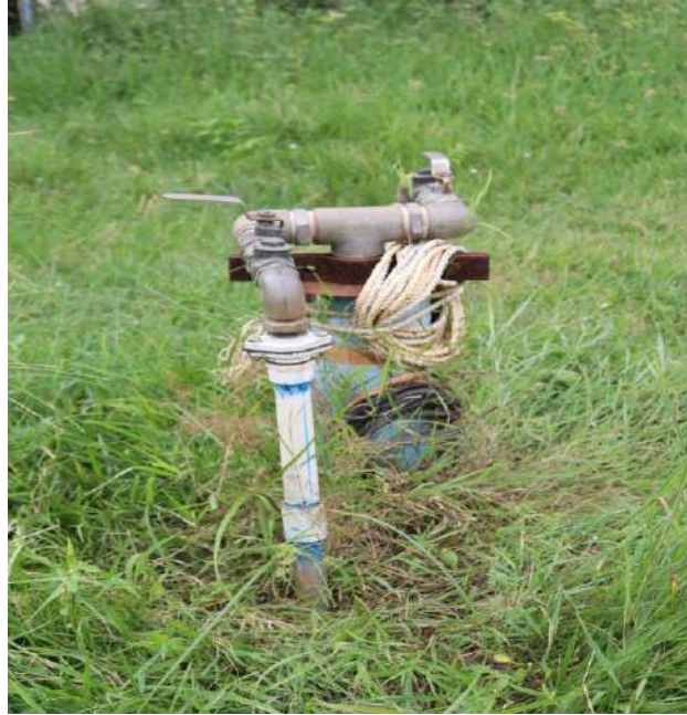
Recharge bore wells on campus
