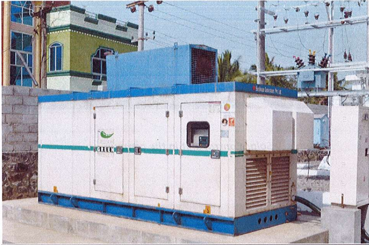
Diesel Generator Inside the Campus
