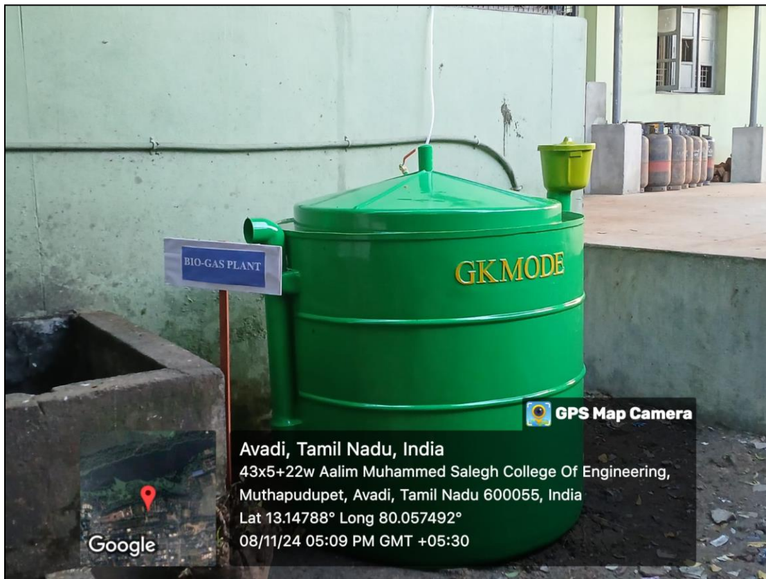
Figure: The Bio-Gas plant Setup installed in the campus
