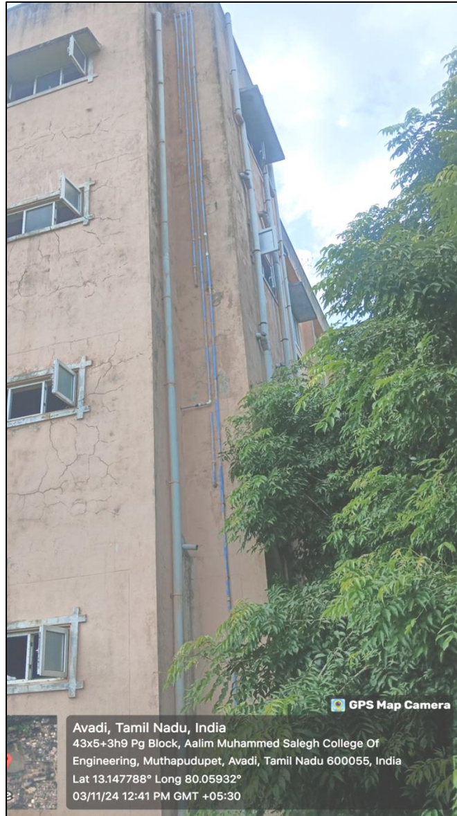
Figure: Water Distribution through Tanks in CSE&IT Block
