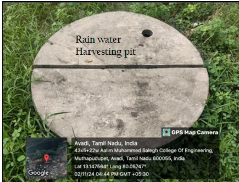
Figure: Rain water harvesting pits near Civil & Mechanical Block
