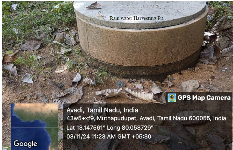
Figure: Rain water harvesting pit in EEE Block
